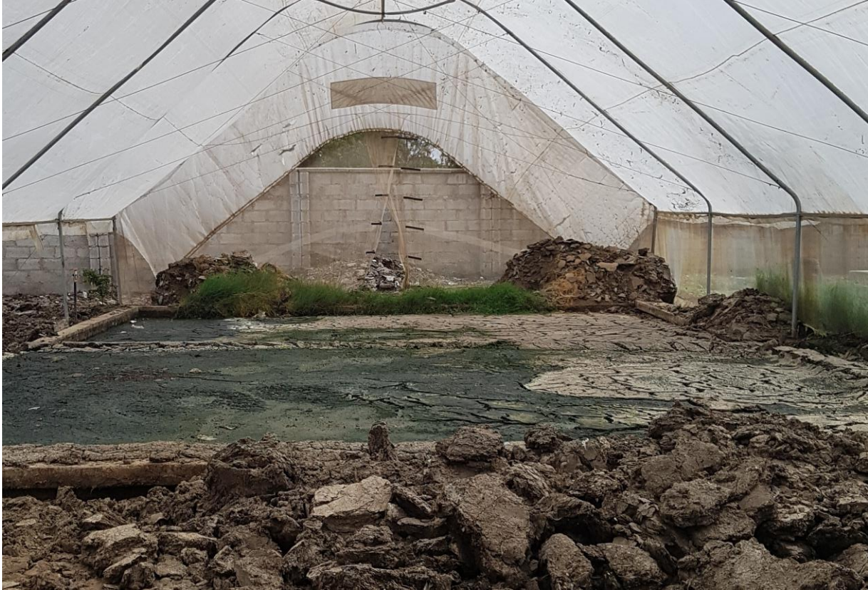
FIGURE 14: SLUDGE DRYING BEDS SERVING AN FSTP IN LUSAKA
