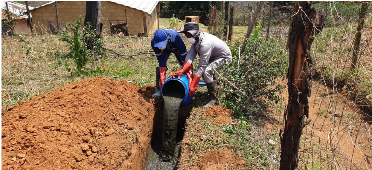
FIGURE 9: ENTRENCHMENT OF PIT SLUDGE IS A SAFE AND ECONOMICAL DISPOSAL OPTION WHICH ELIMINATES THE NEED FOR TRANSPORT IF THERE IS SPACE FOR IT TO BE DONE ON THE SITE WHERE THE PIT IS EMPTIED. ETHEKWINI HAS USED ON-SITE BURIAL FOR MOST OF ITS PIT SLUDGE DISPOSAL. TREES PLANTED OVER OR NEAR THE DISPOSAL SITE SHOW ENHANCED GROWTH.
