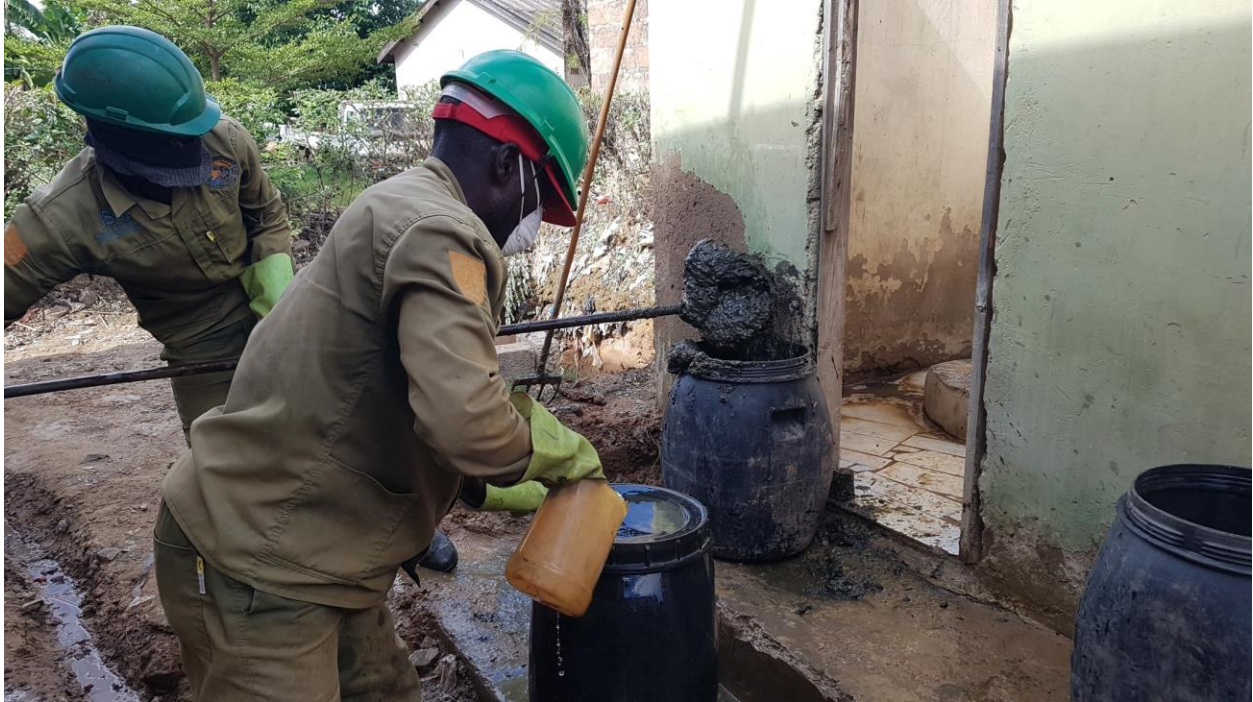
FIGURE 7: MANUAL PIT EMPTYING USING LONG HANDLED FORKS, SHOVELS AND SCOOPS. AFTER COMPLETION THE SITE IS WASHED DOWN WITH A STRONG DISINFECTANT SOLUTION
